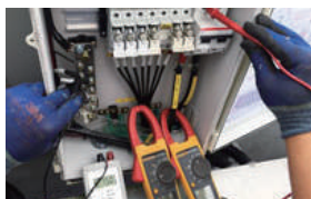
檢查發電 - RA量測 Inspection of Power Generation - RA
