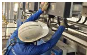
清理INV通風口 Clean for Air Vent of Inverter
