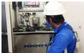
檢查SMP盤 Inspection of SMP
